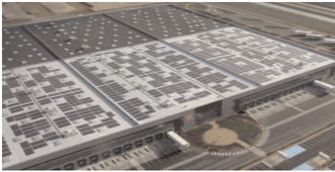
ProLogis Solar Panels Moissey Cramayel, Chanteloup, France
